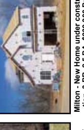
Milton - New Home under construction. 3 BR, 2.5 BA, $239,900 Buy Now & Make It Your Own! #132429H David Bledsoe 304-634-7349
