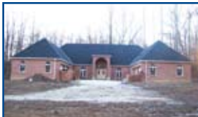
Ashland - Custom built 3-5 BR, 3 BA ranch home w/open floor plan of 4680+/- sq.ft. in Ashland's only gated community. $275,000 #27277 (EAM)
